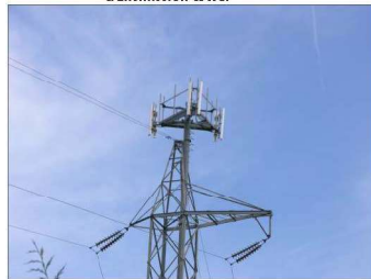
Exhibit 3-1. An antenna array mounted on top of a transmission tower
